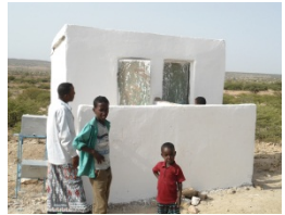
Latrines constructed on Dharar Wahar earth dam under Dila village, the children and their father were very happy to see the latrines when they are using the water of the earth dam
