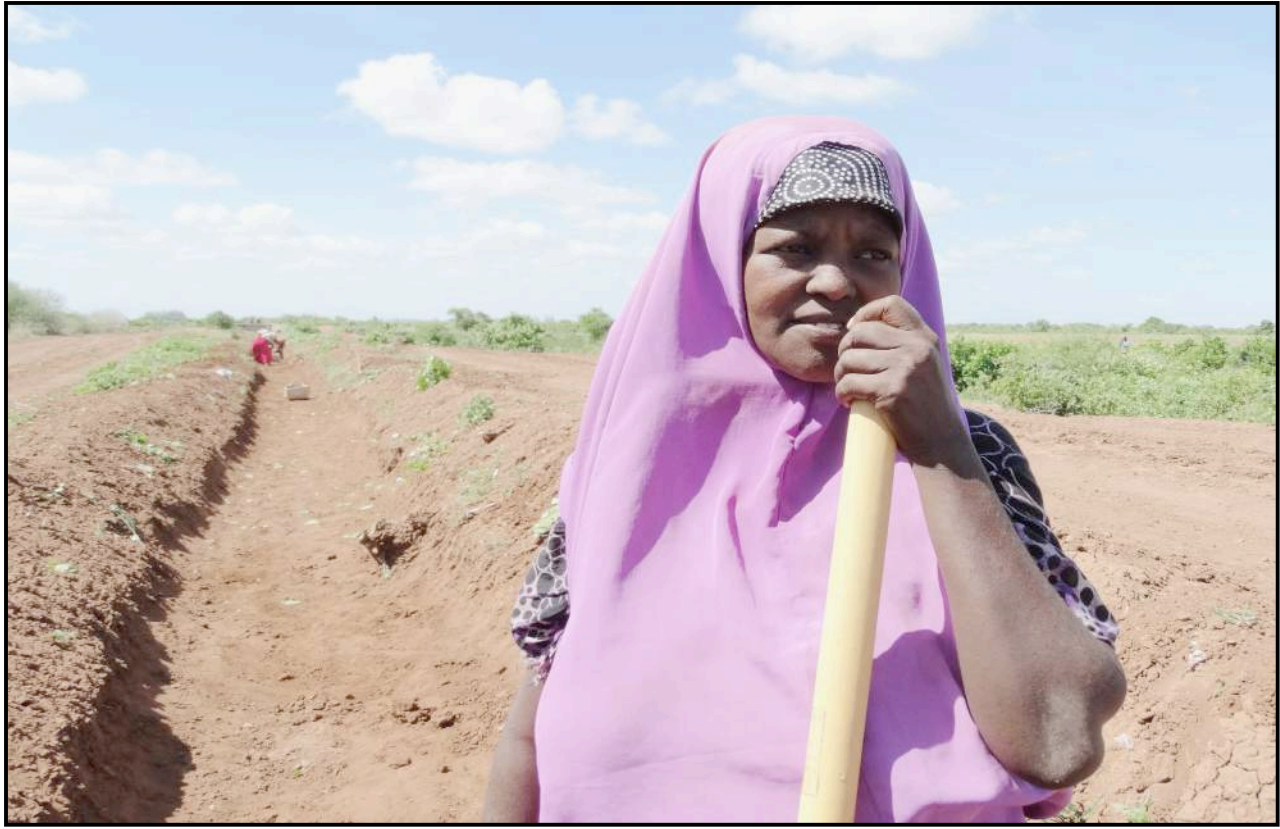
Fama Hussein Shiqow of Raqayle village at the canal rehabilitation site, Afgoye District
