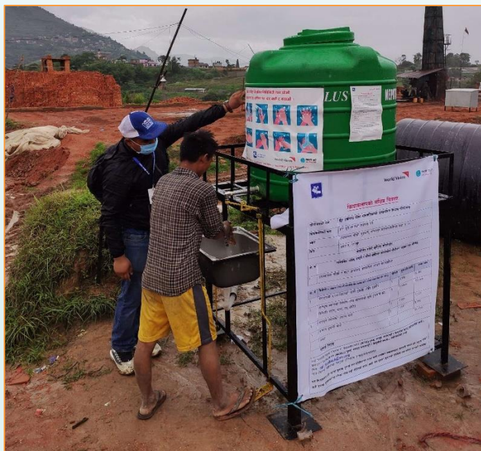
Fig 2: Hand washing station installed by WVI Nepal in a Brick industry in Kathmandu
