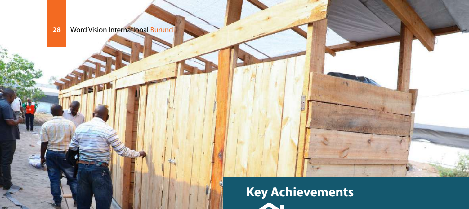
WVIB has built a block of 16 latrines for internal displaced people from Gatumba at Kinyinya I, Mutimbuzi Commune
